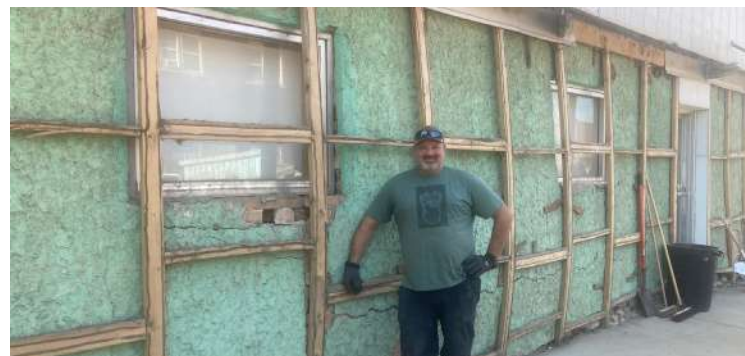
Owner Sam Silacci stands along the exposed east wall of Dakota Territory Arms building, formerly the Cliff Thomas Drugstore. Demolition was in part, funded by a grant from Outside of Deadwood Historical Preservation. Beacon photo
