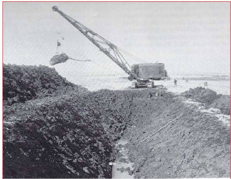
After the inspection of 1924, of the drainage problem on the Irrigation Project, the drain ditches were dug all over the Project. Newell Museum
